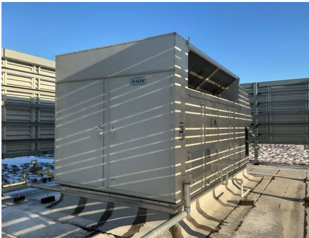
15 - ROOFTOP HVAC UNIT
